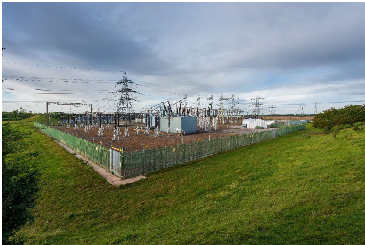
Figure 3.8 - Typical substation (existing Monk Fryston Substation)
